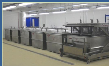
CAHID's new mortuary houses specially designed equipment for Thiel embalming
